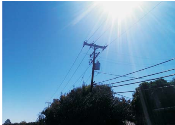
Photograph 8: View of the pole-mounted transformer on the southern boundary of the subject property, facing southeast.
