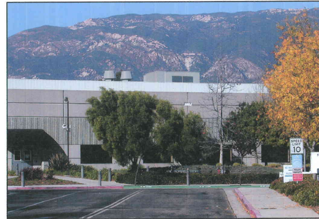
PROPOSED FRONT OF BUILDING WITH NEW MECHANICAL SCREEN AND PAINTING OF AH & EF
