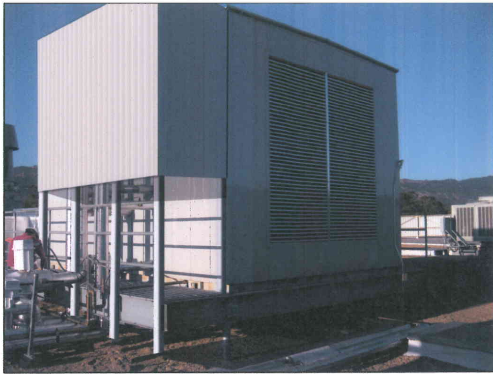
NEW MECHANICAL SCREEN AT AIR HANDLER
