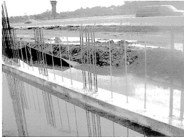
Figure 7: Failing BMPs at a Cal Trans construction site on Hwy 101.
