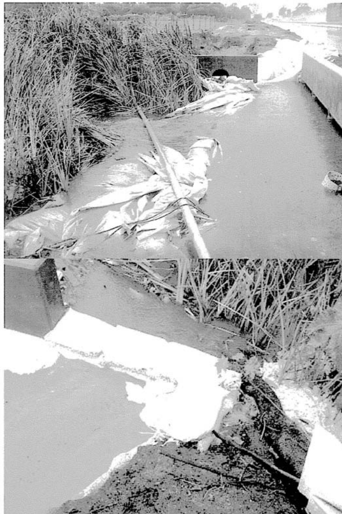
Figure 5 and 6: Breached construction site BMPs carrying suspended sediments into Santa Barbara Bird Lagoon
