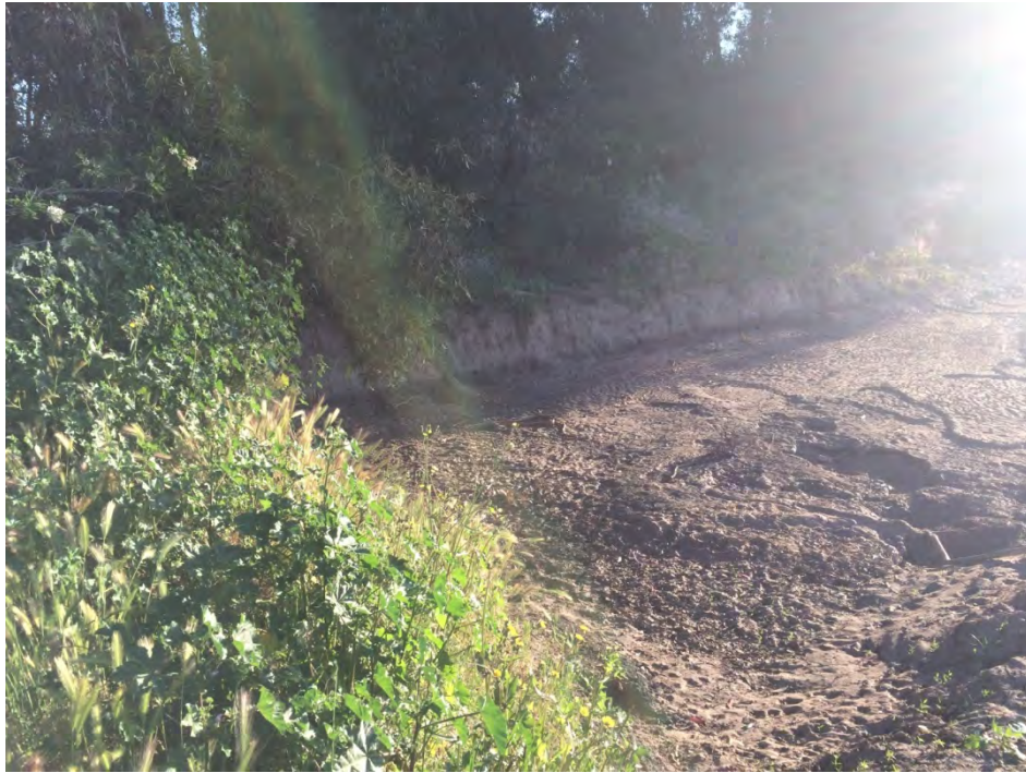
Photograph 1. Close up view of western end of proposed restoration site, view facing northeast. Construction site at the time of photo. Old San Jose Creek channel not visible, located to the left/north. April 20, 2017
