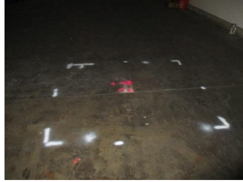
GPR investigation of pipes in the floor in the southwest corner of the west warehouse space.
