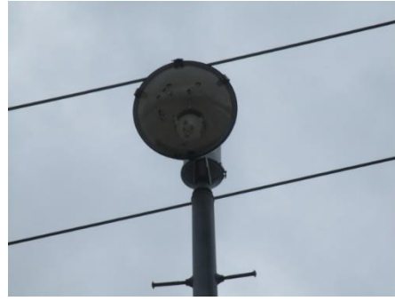
Unidentified exterior light type on pole.
