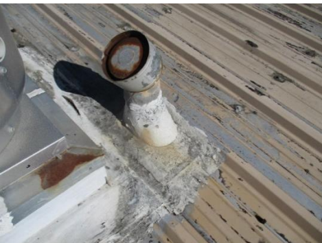
Asbestos containing transite flue on roof.
