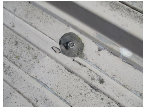
Asbestos containing roof tar sealing bolts penetrating the roof.
