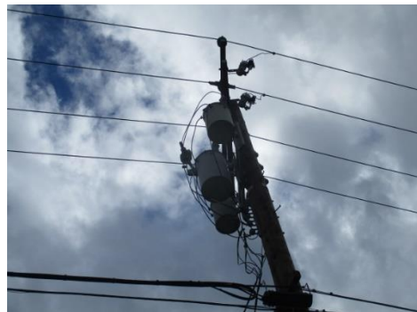
Pole-mounted transformers along the south subject property border.
