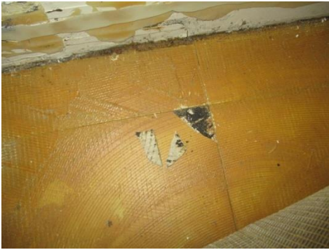
Asbestos containing black floor mastic and floor tile contaminated with the mastic.
