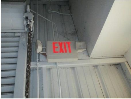
Typical battery powered exit sign and emergency lights.
