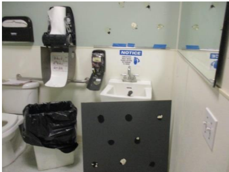
Asbestos containing mirror mastic.
