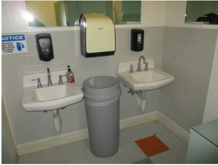
Lead-laden ceramic wall trim in the men's bathroom behind and next to sinks.
