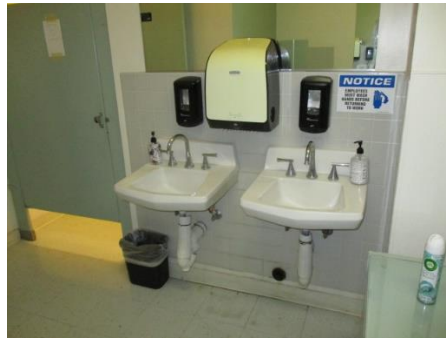
Lead-laden ceramic wall trim in the woman's bathroom behind and next to sinks.
