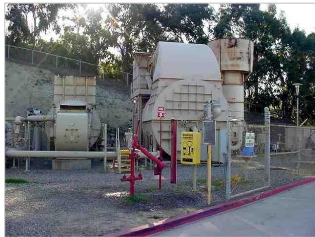
Oil Processing Equipment at the Venoco Ellwood Onshore Oil Gas and Processing Facility
