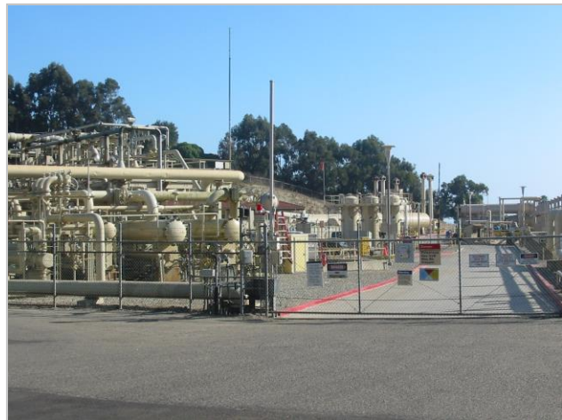
Processing Equipment at the Venoco Ellwood Onshore Oil and Gas Processing Facility
