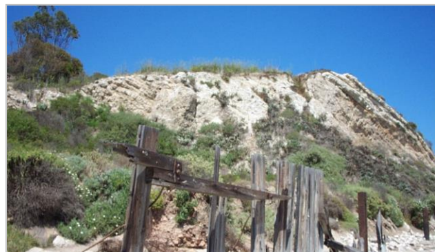
Remnants of Seawall at the Base of the Ellwood Mesa Bluffs
