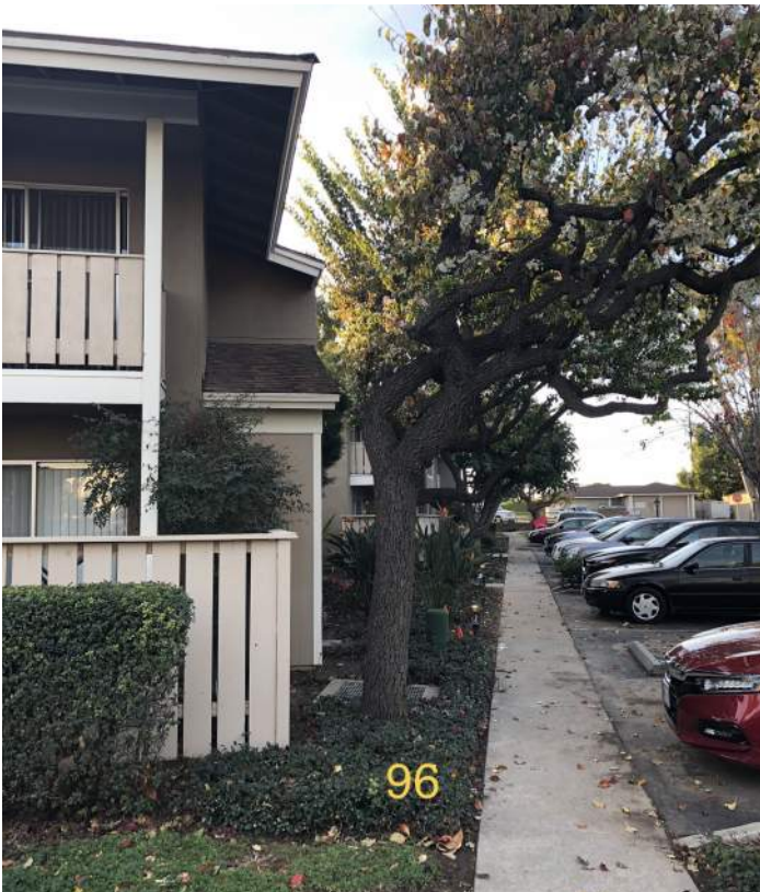
Several of the pears are severely topped and pruned to keep the crown away from the building eaves. These trees are mature and will require extensive maintenance to maintain this form into the future.
