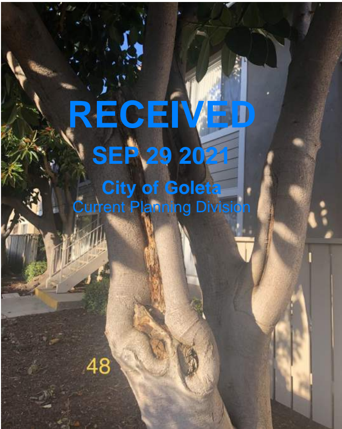
This is a typical image of the exposed heartwood and visible decay present on the rubber trees onsite. This damage likely stems from a long history of overpruning to maintain the small size they exist in today.
