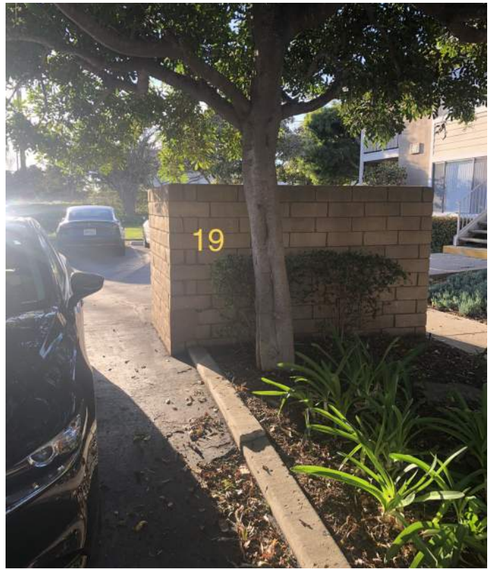
Typical example of AC pavement upheaval and curb damage from underground surface roots.
