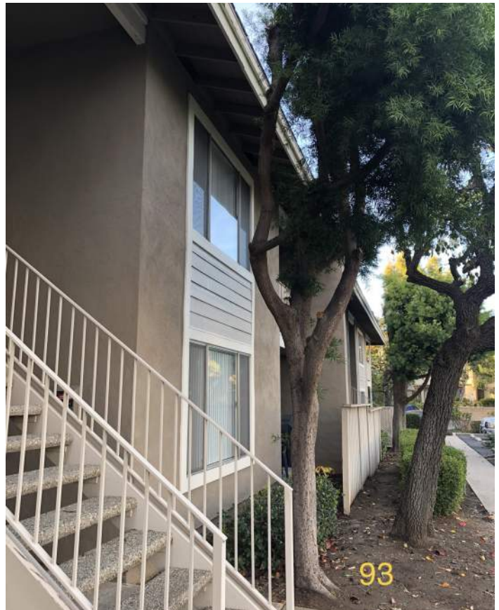
This image represents a the typical planting conditions of the African fern pines observed onsite. Many are severely crowded by adjacent structures and should be replaced further from the structures (or elsewhere onsite) with a suitably sized species.
