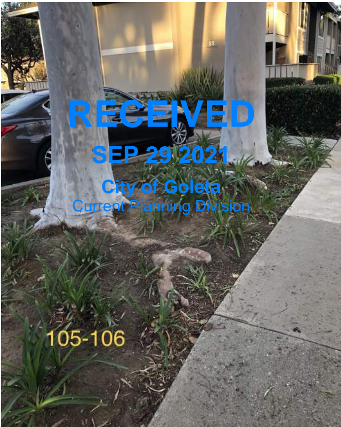
This image shows evidence of root pruning on these stressed lemon scented gums. It's likely the roots damaged the paving, and the paving contractor removed the surface roots to repour the pavement in place.
