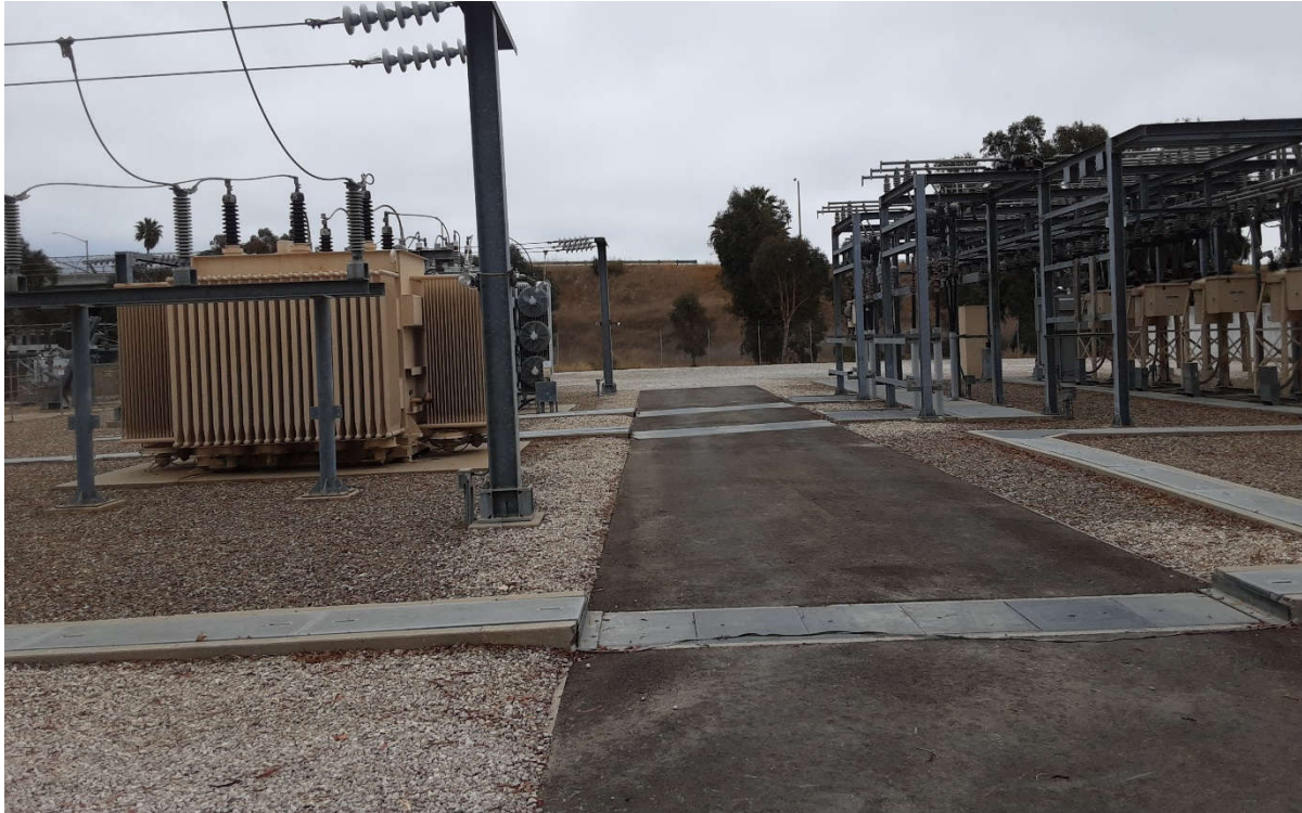
Photograph 5. View of substation facing east.
