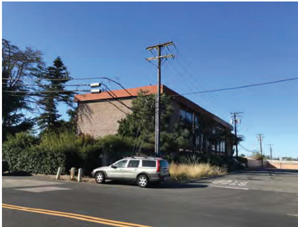
Photograph 11. View of the southern adjacent commercial office building and pole-mounted transformers (33 S. La Patera Lane), facing southwest.
