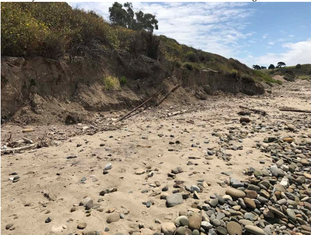
Photo 10. Westerly view looking toward Bell Canyon Creek mouth showing eroded bluff face with old exposed pipes.
