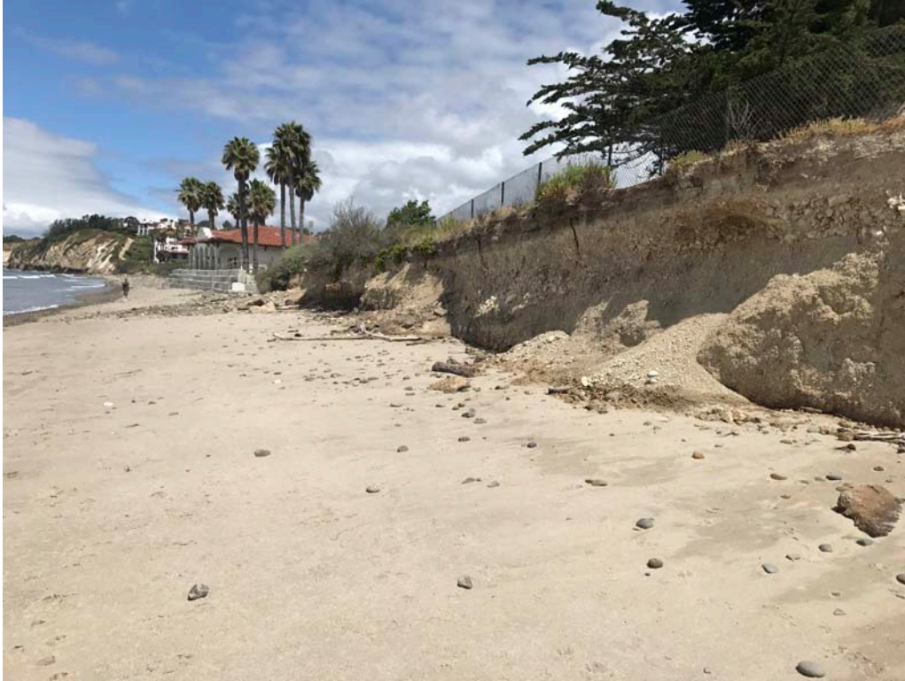
Photo 9. Westerly view of eroded bluff face below trail. Note fence near edge of bluff.
