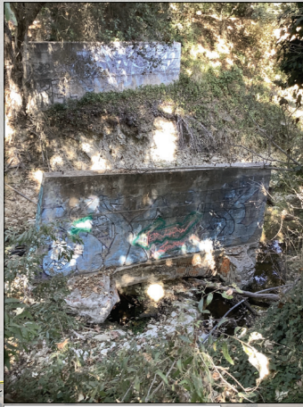
Abandoned bridge abutment in channel bed
