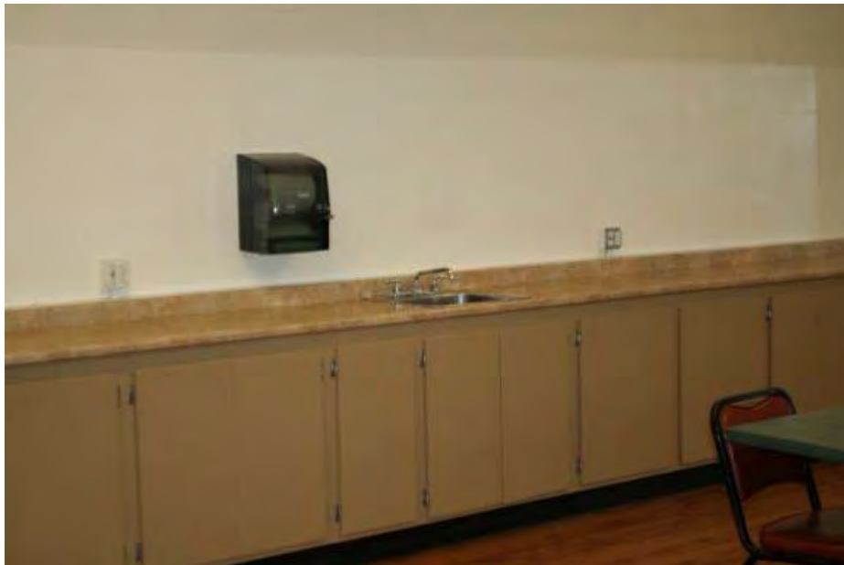
Figure 8 – Building A, non-compliant cabinet and sink
