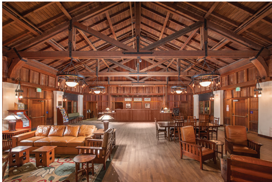
Figure 21. Sensitive installation of fire sprinkler and seismic reinforcement in architecturally significant interior spaces.
