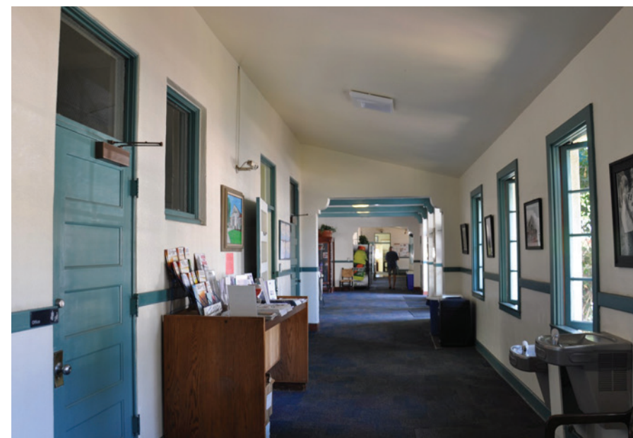
Figure 16. Wood paneled doors and corridors are character-defining features that can be adapted with ADA-compliant hardware.
