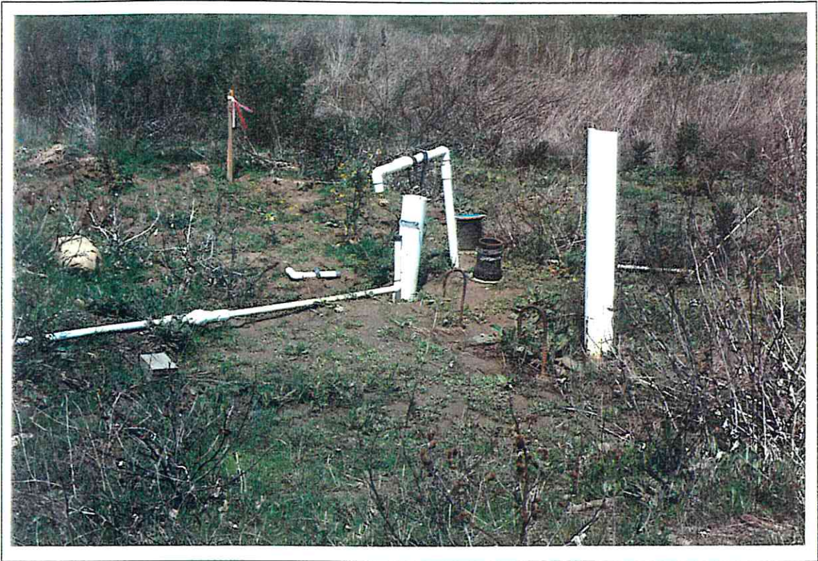
Photo 3. Newer water well on south of site.
