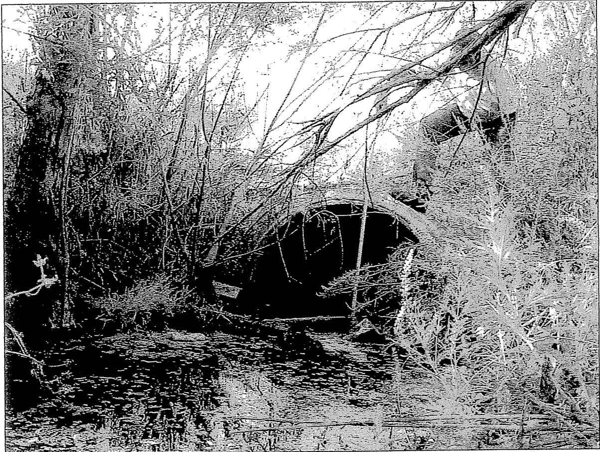
Figure 3-Whittier Drive Storm Drain Discharge Point. The author is using a tape measure to collect measurements of the usable space in the pipe. The discharge pipe is a circular reinforced concrete pipe with a diameter horizontally of 5-feet. The pipe has significant sediment below the water line because the depth to sediment from the top of the pipe is only 3 feet.
