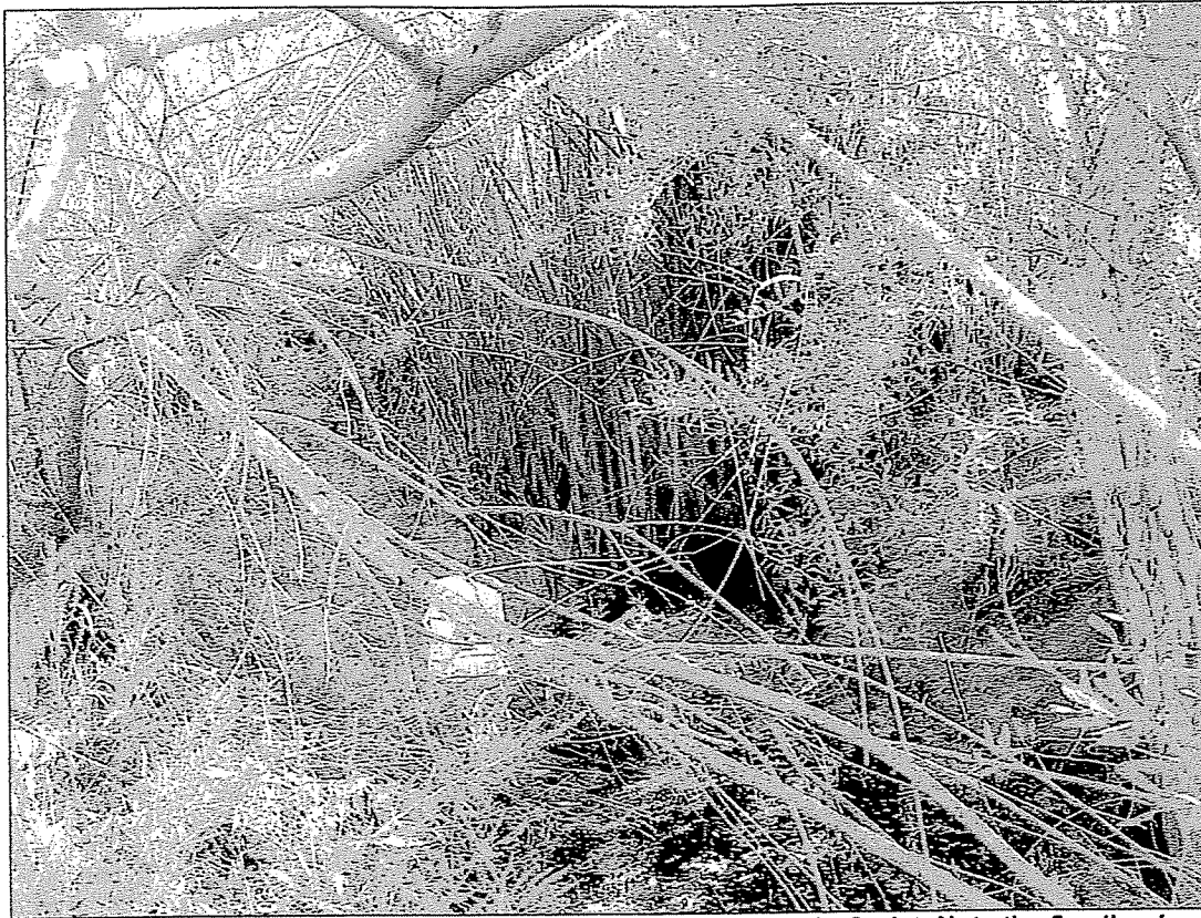
Figure 4-Open Channel downstream from Whittier Drive Storm Drain Outlet. Note the 5-gallon bucket for scale. The channel is so heavily vegetated its difficult to locate the bucket. There is a wall of vegetation even thicker behind the bucket.
