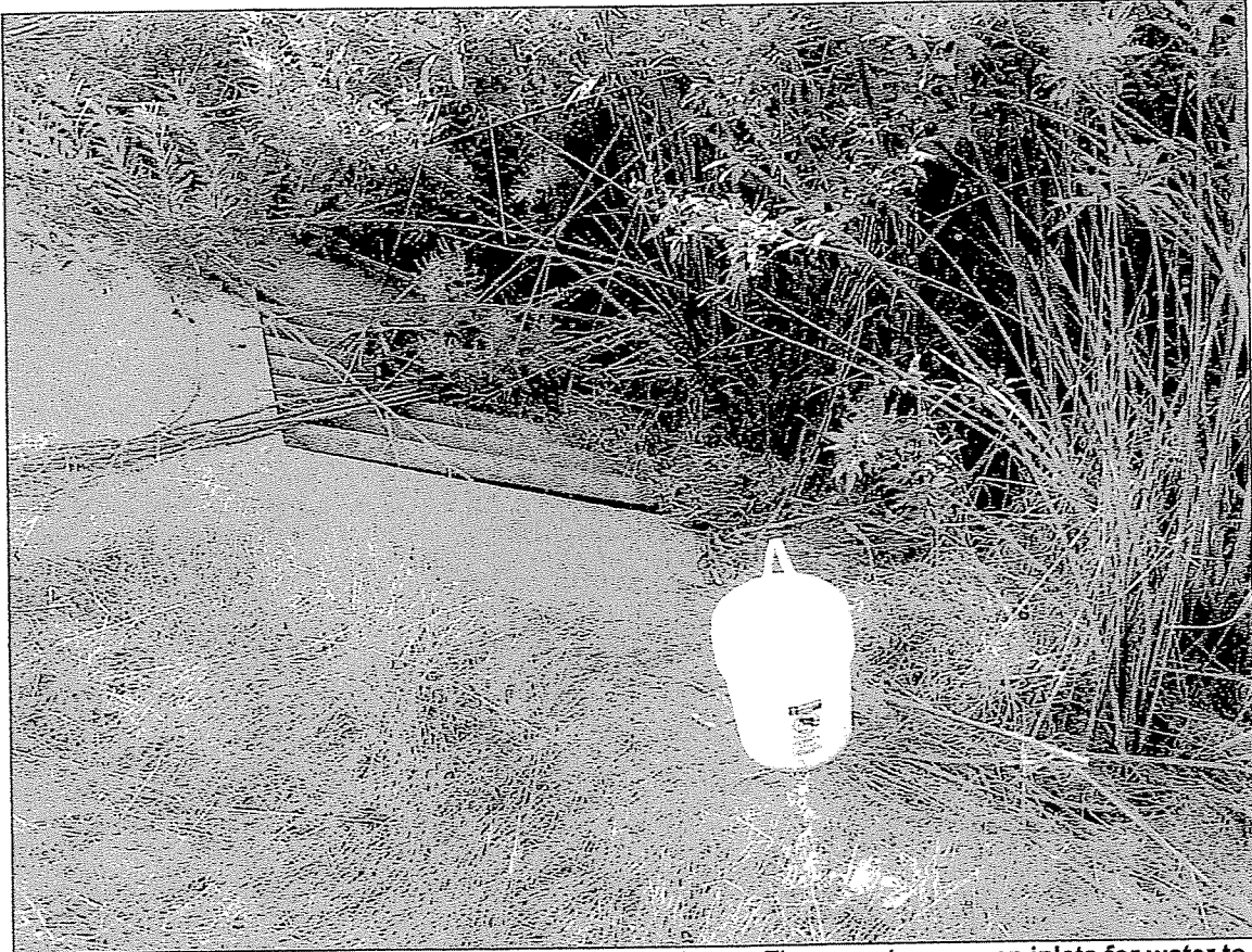
Figure 2-Biofiltration Basin shows the heavily wooded area. There are two screen inlets for water to enter the storm drain that drains the area. There is an upper grate to the left of the photo and a lower grate. Note the clogging of the lower grate by heavy vegetation. Note the 5-gallon bucket for scale.
