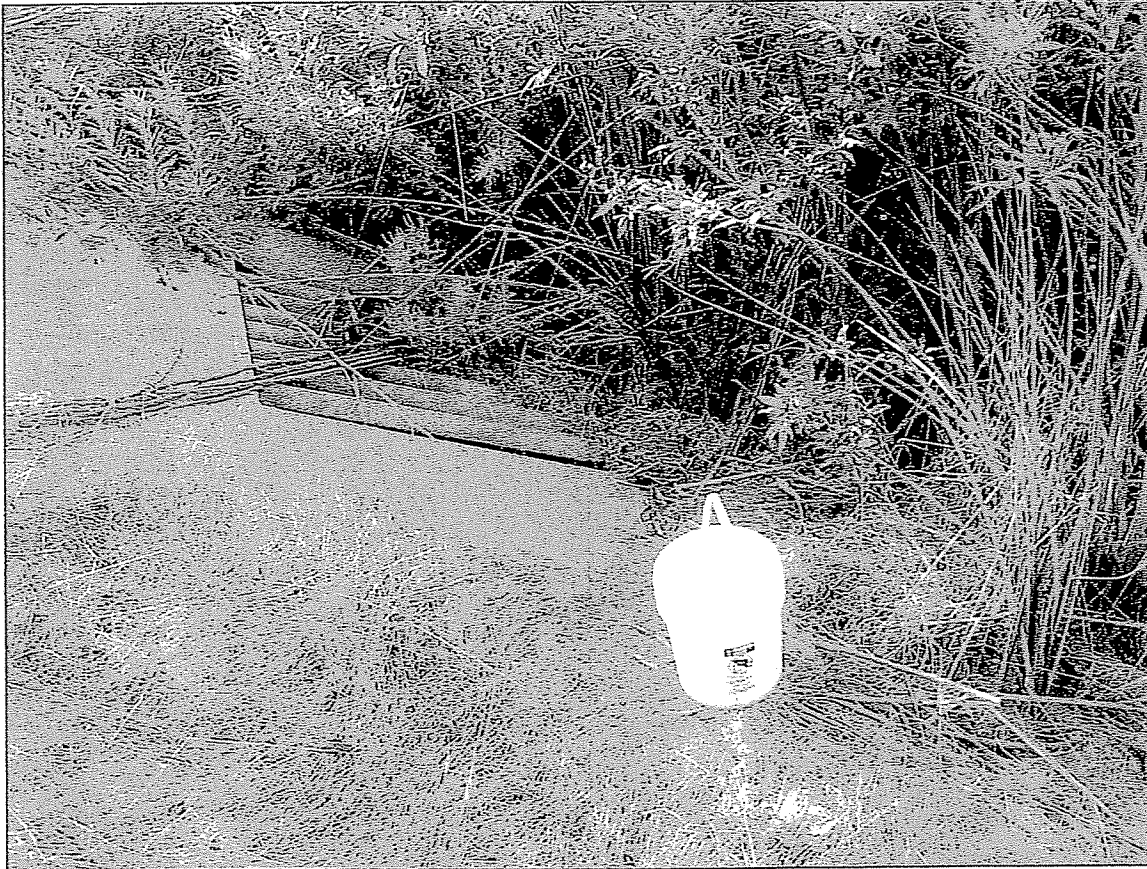
Figure 2-Biofiltration Basin shows the heavily wooded area. There are two screen inlets for water to enter the storm drain that drains the area. There is an upper grate to the left of the photo and a lower grate. Note the clogging of the lower grate by heavy vegetation. Note the 5-gallon bucket for scale.
