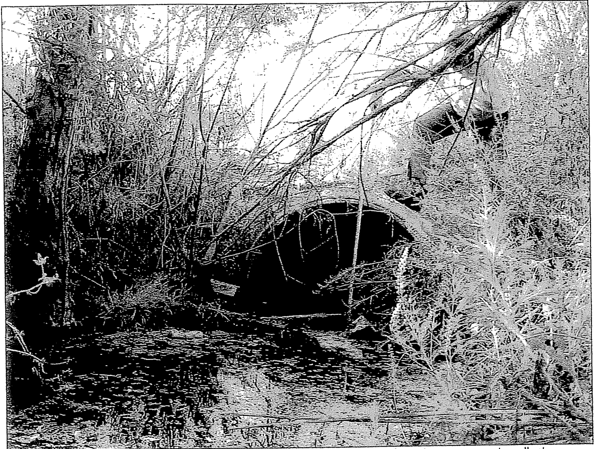
Figure 3-Whittier Drive Storm Drain Discharge Point. The author is using a tape measure to collect measurements of the usable space in the pipe. The discharge pipe is a circular reinforced concrete pipe with a diameter horizontally of 5-feet. The pipe has significant sediment below the water line because the depth to sediment from the top of the pipe is only 3 feet.
