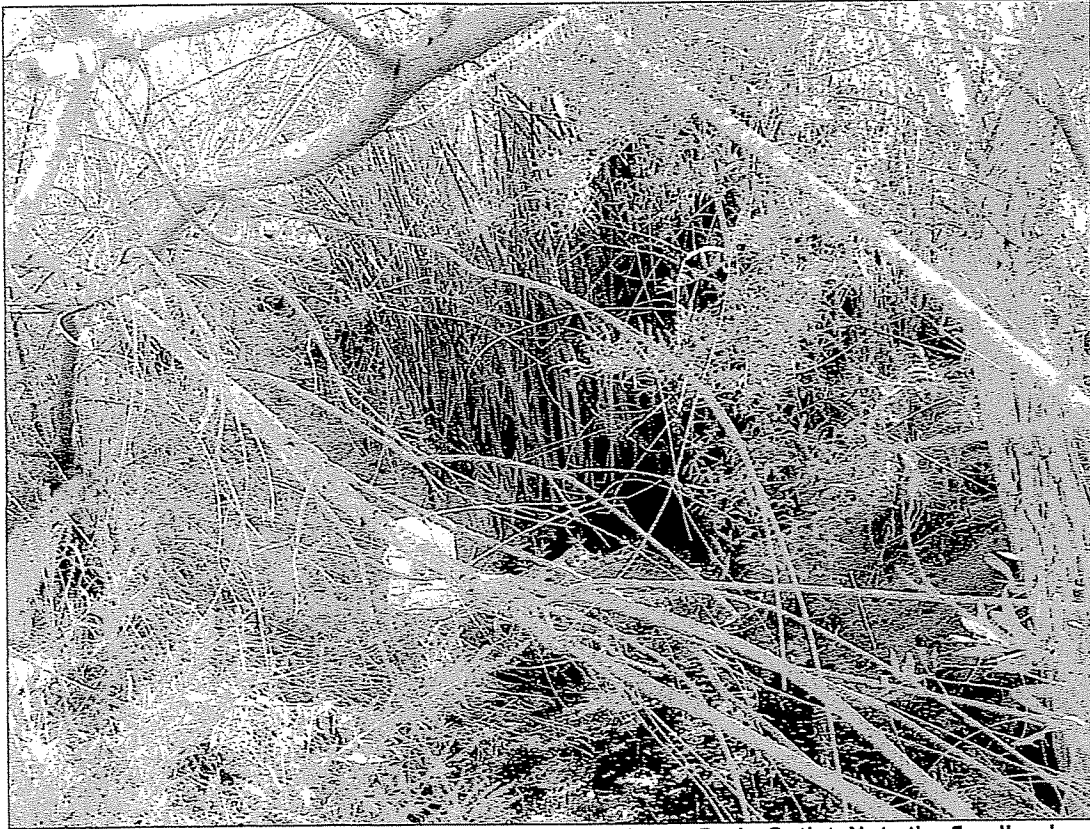
Figure 4-Open Channel downstream from Whittier Drive Storm Drain Outlet. Note the 5-gallon bucket for scale. The channel is so heavily vegetated its difficult to locate the bucket. There is a wall of vegetation even thicker behind the bucket.
